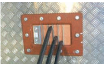
• Bolted transit for power cables
