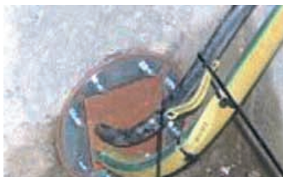
• RGP-transit enclosed in the power base.
