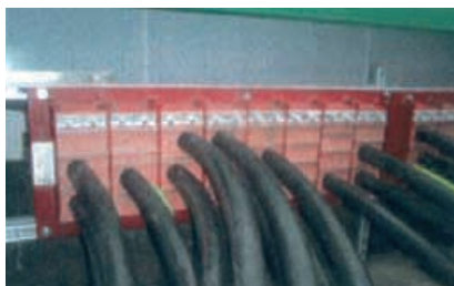
• Cable routing from the tower to transformer room
